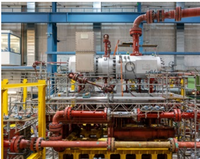
Heat pump unit on the test bed
